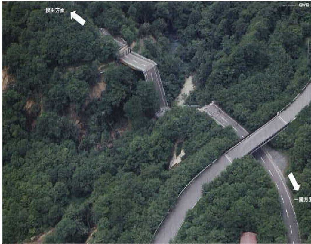
Fall of Bridge Girder due to Movement of Foundation caused by Slope Failure
