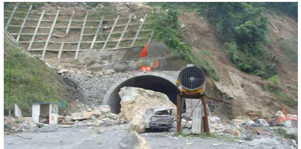
The place of reinforced slope (frame) suffered only slight damage. 20
